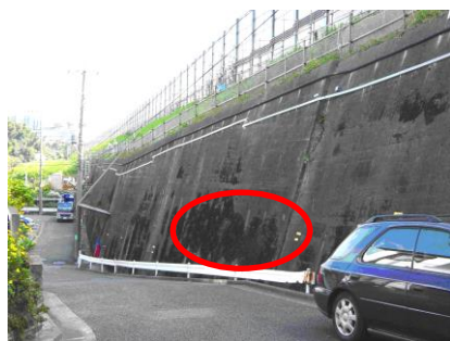
道路法面背面空隙
