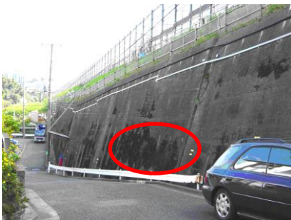
道路法面背面空隙
